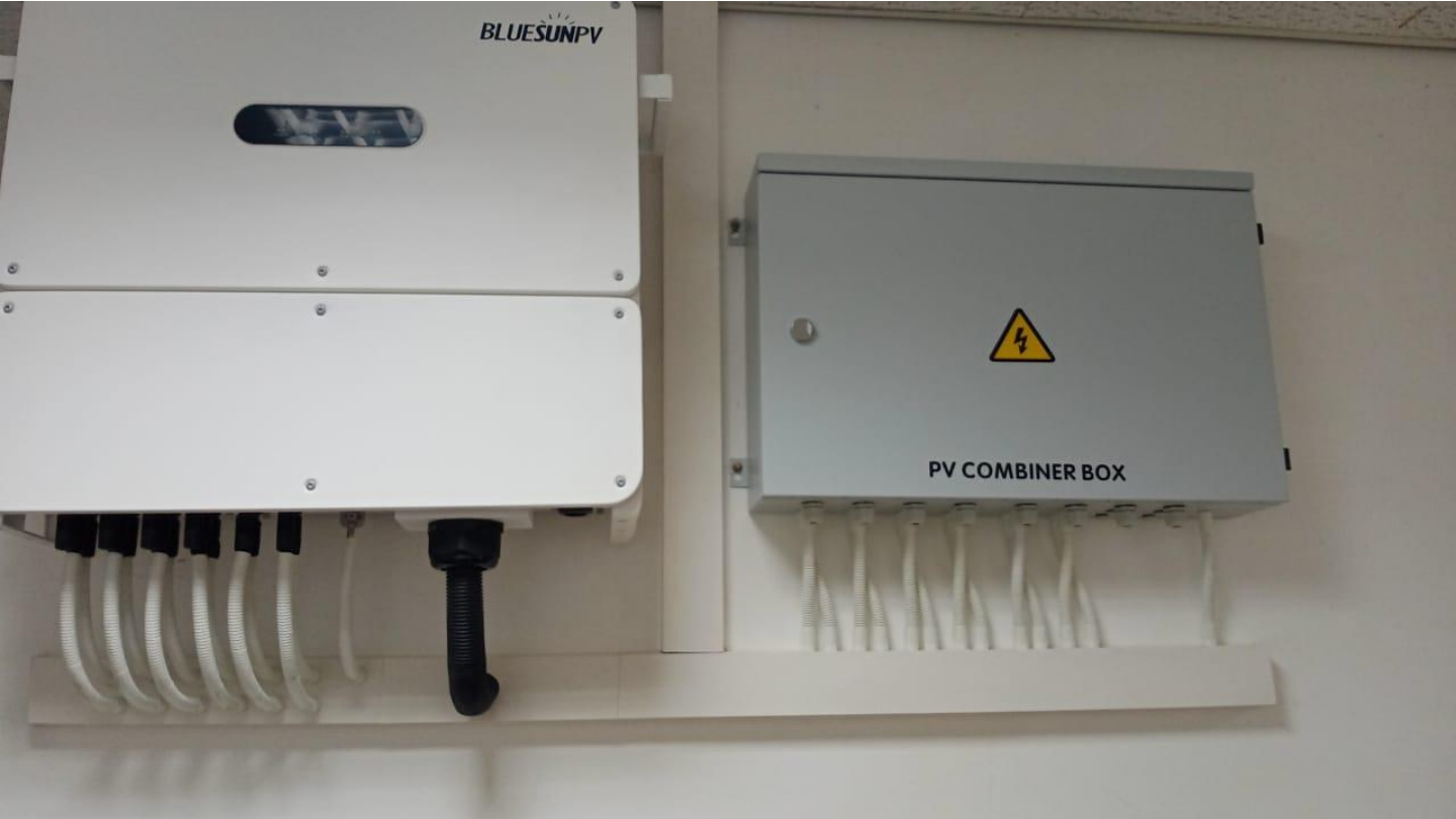
Figure 8 Photo of Inverter and PV Combiner box
