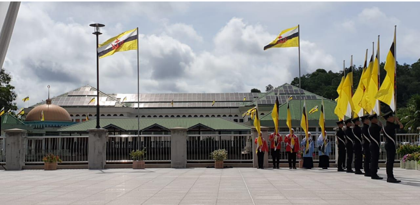
Figure 9 Photo of 100kW Solar PV System installed on the rooftop of Temburong District Office
