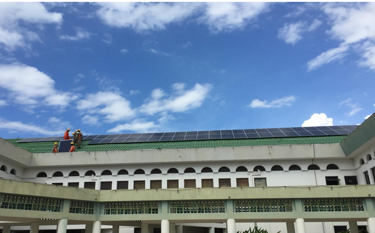
Figure 1 Solar panels installed at the rooftop of a building
